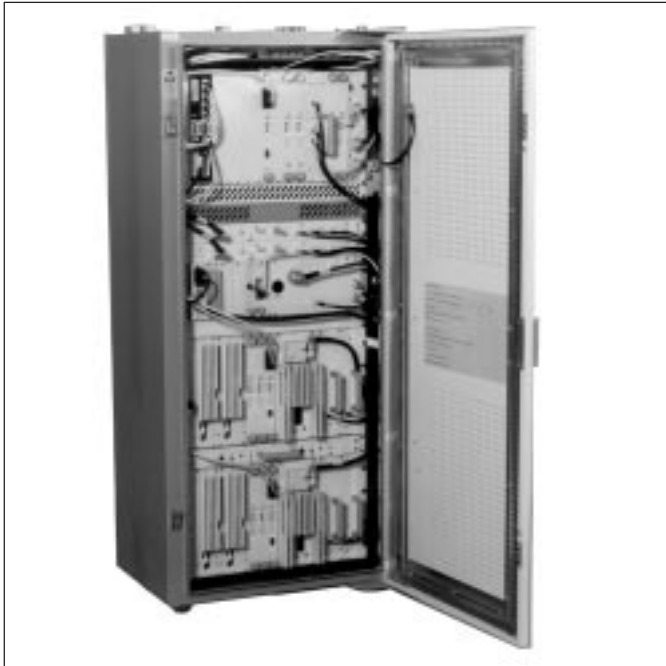
Base station of cellular network
